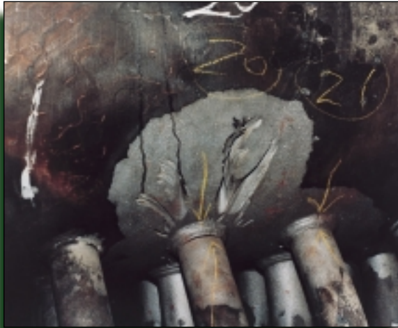
Figure 1: Photo of header where metal was removed by the washing action of steam leaks — a result of undetected ligament cracks.
