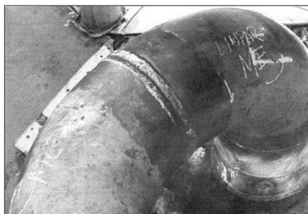
10. Preparation for non-destructive testing (ultrasonic and magnetic particles) of a crossover pipe welding.
