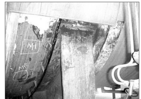
8. Preparation for inspection and non-destructive testing in the deaerator tank saddle. Simultaneously, the vessel itself had been tested internally by wet fluorescent magnetic particles.
