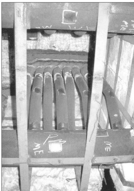
3. Access provided for inspection of elements in the interior of penthouse and other "cold" chambers in the recovery boiler.
