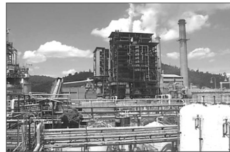
13. CENIBRA’s recovery boiler No. 1. This unit had its first start-up in 1977, and underwent an integrity evaluation program in 2002, according to the guidelines described in this paper.
