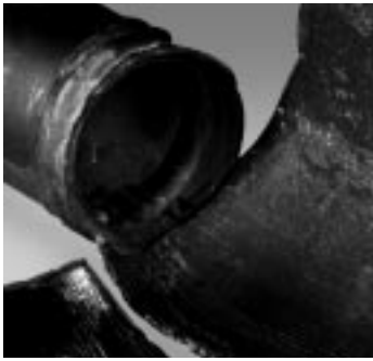
Failure of carbon steel tube at butt weld
