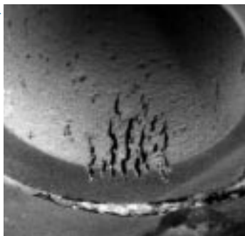
Corrosion fatigue on tube ID adjacent to attachment
